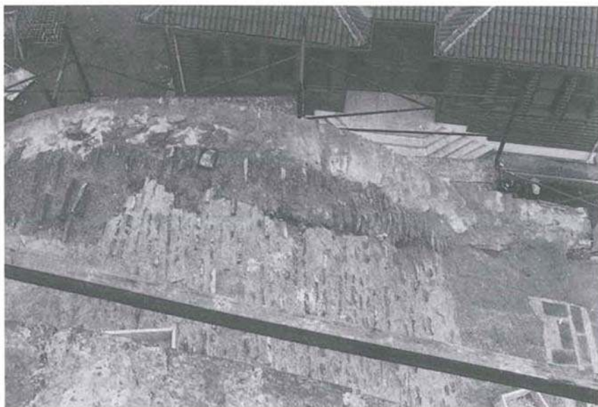
Figure 4. Zeyrek Camii, north church, crack on the vaulting of the northern crossarm (A. Neftçi, 1997).
